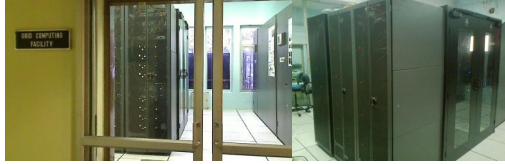
FIG. 2: Grid Computing Facility after Cold aisle Containment implementation
